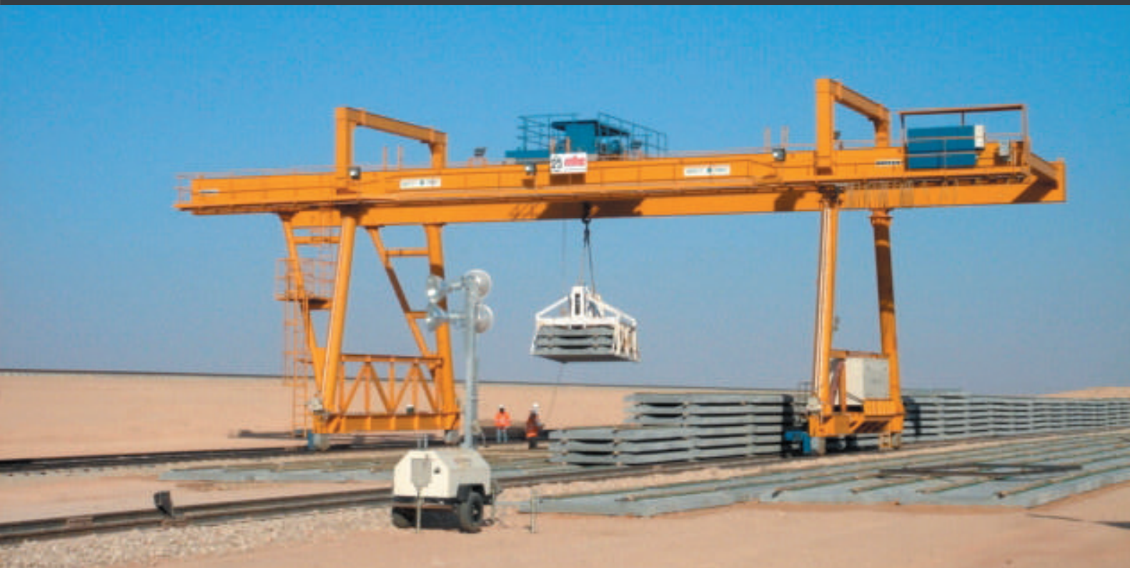
Gantry for Sleepers loading
